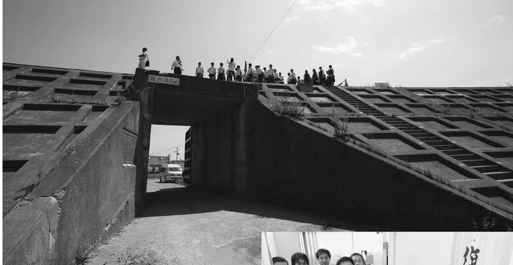
Above: Seawall built at Tarō following the 1933 Shōwa Sanriku Tsunami. It was insufficient to stop the tsunami caused by the 2011 Great East Japan Earthquake.
